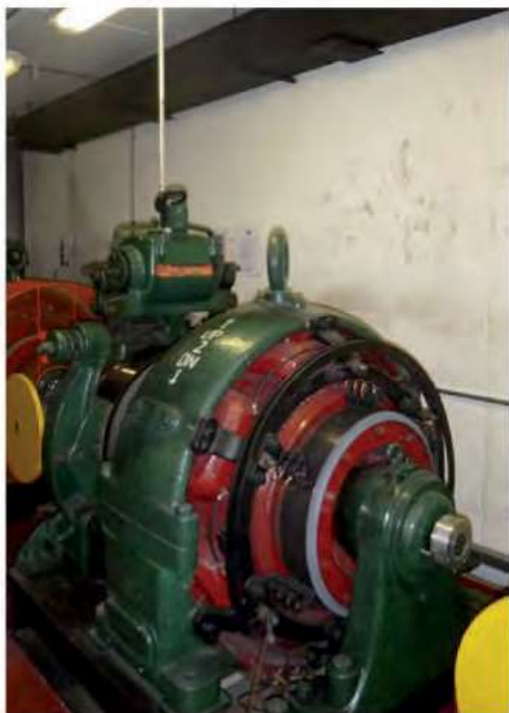
Original lift machine
