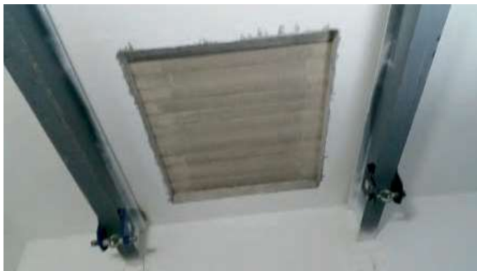
A cutout was made in the machine-room roof for lift machine transportation to the machine room by using a tower crane. Runway beams were fixed below the slab for installation and future repair or modernization, or full machine replacement.
