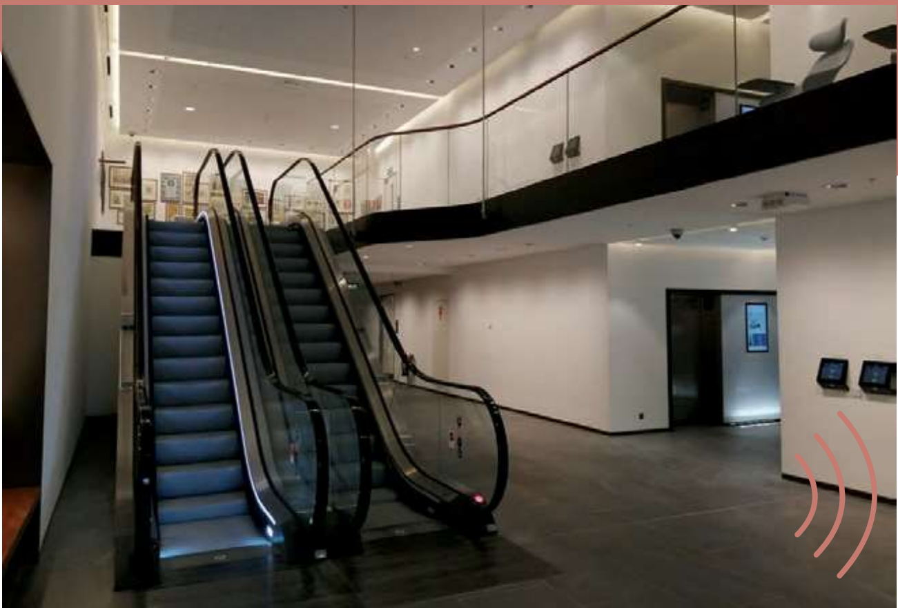
Escalators take building tenants and visitors up to the new mezzanine, which provides access to the upper decks of the new double-decker lifts.
